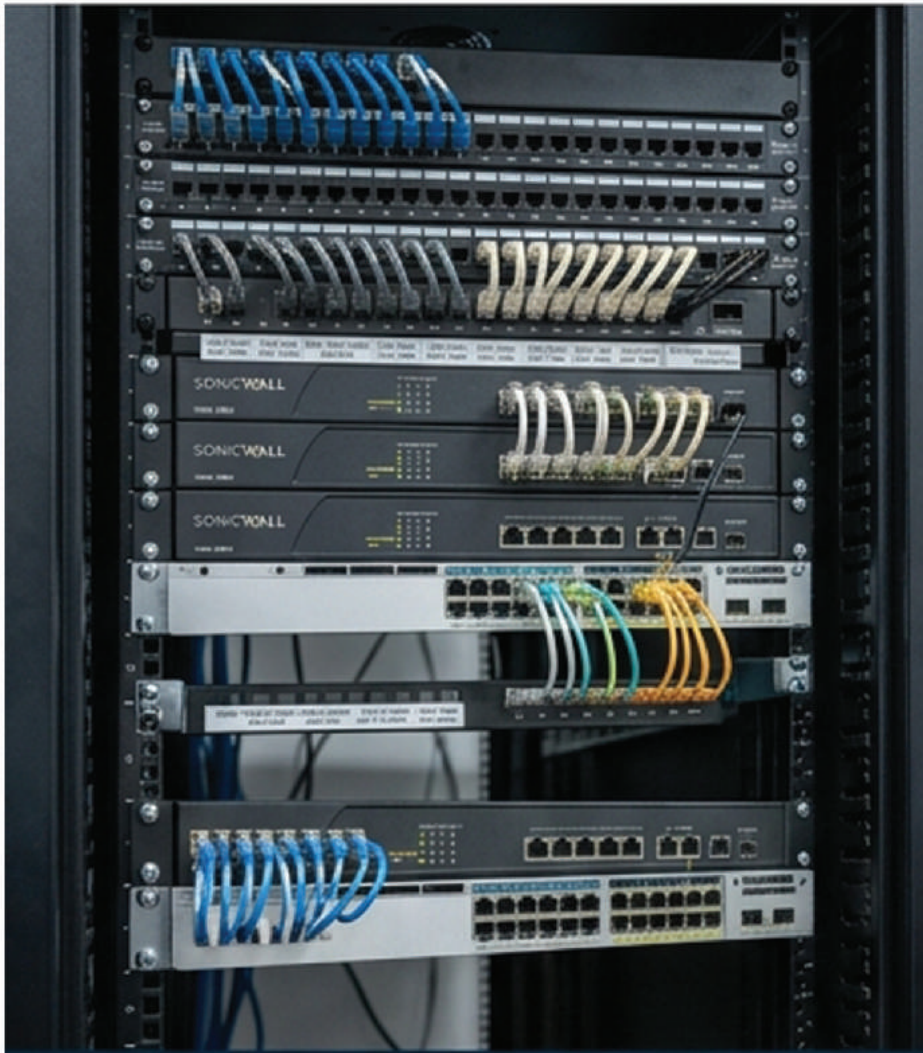
1. Rack-mount build with a rack-mount Firewall. Scope: mounted rack and managed switch.
